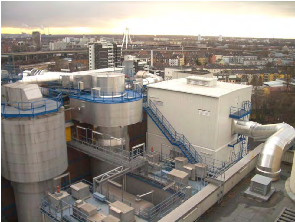
Pic. 13: Spray absorber head and filter / reactor building
